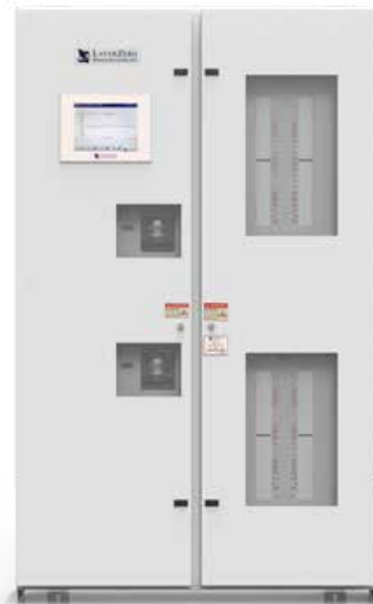
Polycarbonate Windows allow Circuit Breaker Positions to be Viewed with the Outer Doors Closed for Main and Branch Circuit Breakers
